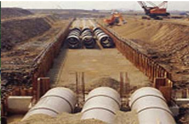
2 Water Distribution System
