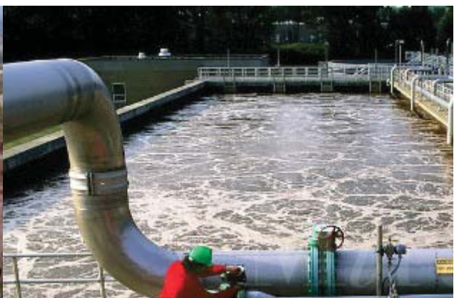
4 Sewage Treatment Plant
